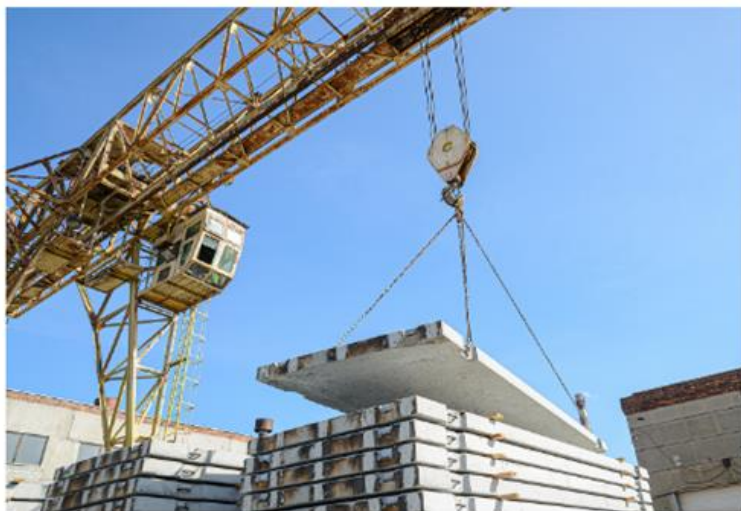
A crane moves reinforced concrete road slabs in a factory warehouse. Image via Shutterstock/Alexandre.ekb.
