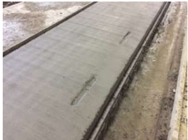
Figure 16. Halfen profiles embedded in the panels for in situ fixing to vertical steel plates
