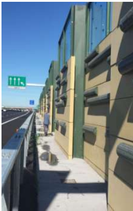
Figure 30. View of installed barrier with upper glass Vista di barriere con vetri superiori
