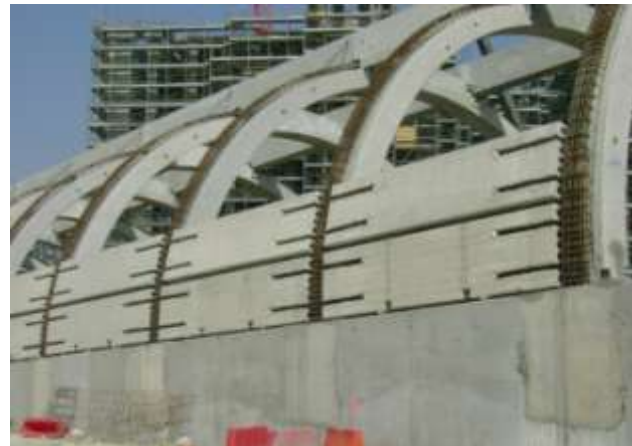
Figure 8. Erection of H C slabs with curved intradox on arches Posa delle lastre ad intradosso curvo sugli archi
