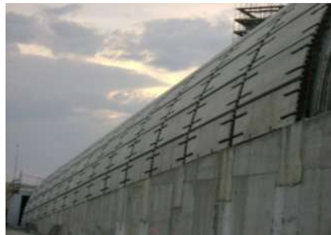
Figure 9. HC slabs positioned to realize the vault of tunnel Lastre posate a secco a realizzare la volta del tunnel
