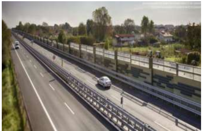
Figure 32. View of completed noise barrier in High-way A4 access Vista di barriera completata in autostrada A4
