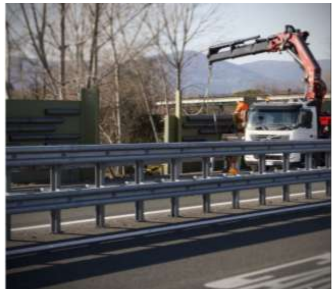
Figure 27. Barriers installation operating from the side lane Posa in opera delle barriere operando dalla corsia laterale
