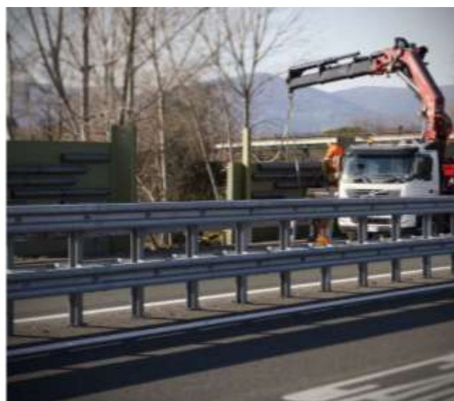
Figure 27. Barriers installation operating from the side lane Posa in opera delle barriere operando dalla corsia laterale
