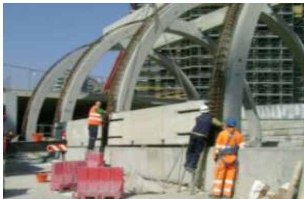
Figure 6. Erection of curved HC slabs for the vault Posa delle lastre curve per realizzare la volta
