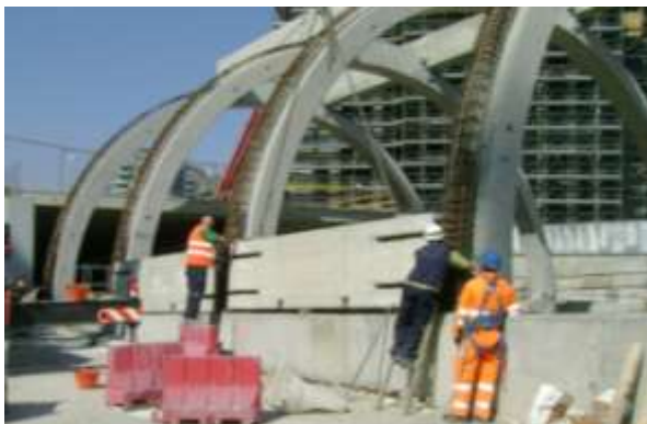
Figure 6. Erection of curved HC slabs for the vault Posa delle lastre curve per realizzare la volta
