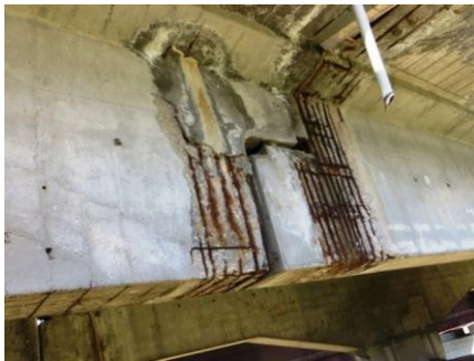
Figure 9: Damage areas close to cantilever girder /ammaloramento delle selle gerber.
